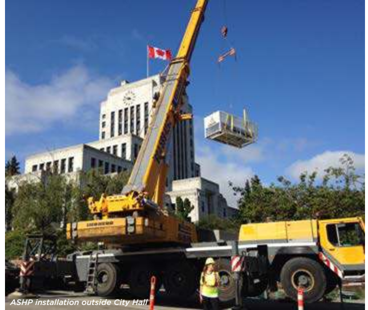
ASHP installation outside City Hall
