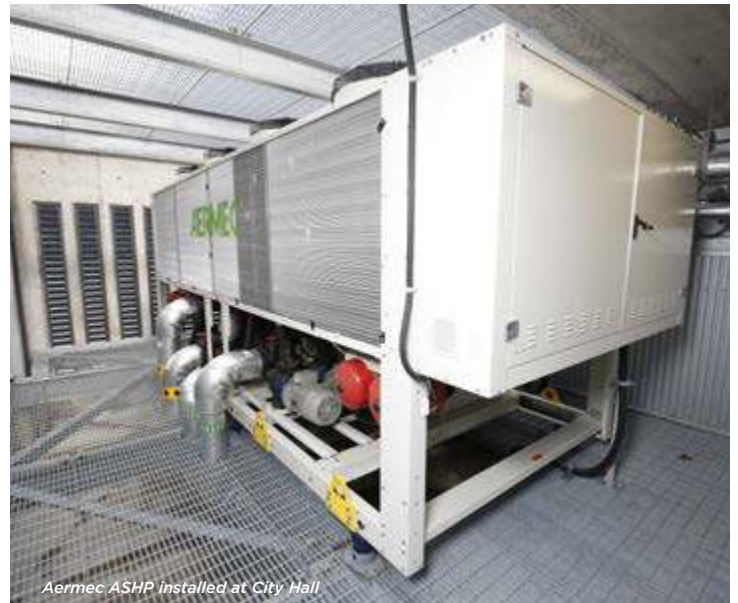
Aermec ASHP installed at City Hall
